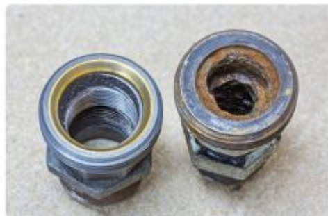
Scale in old pipe after years of using
