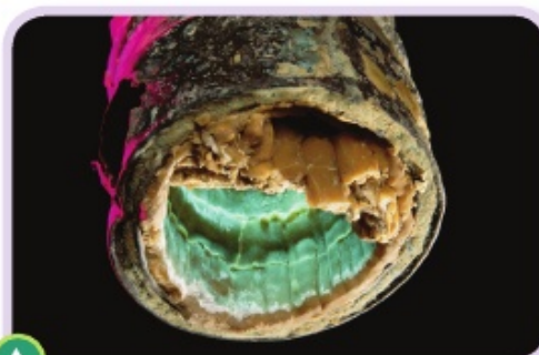
Figure 10.15 Thick deposits of limescale on the interior of a hot water pipe
