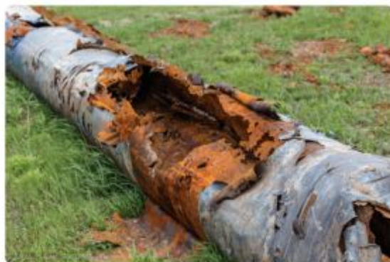
Corroded old large water pipes after many years of uses
