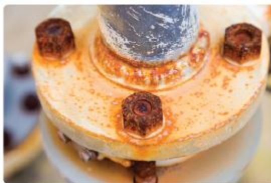
Corrosion is slow process
