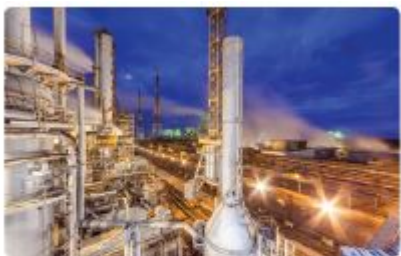
Nitric acid production on fertilizer plant
