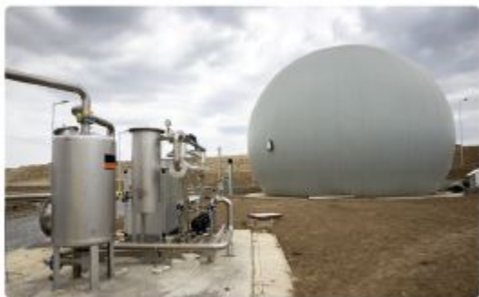
Natural gas tank
