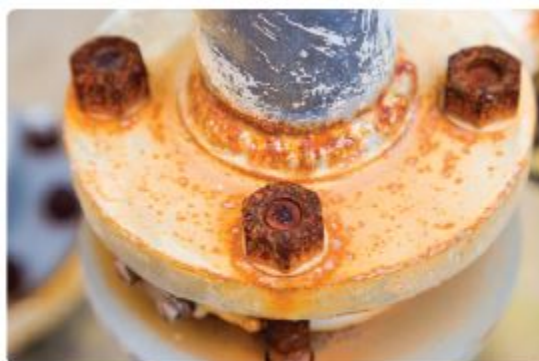
Corrosion is slow process
