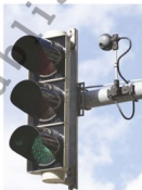
8.5 Traffic light with sensor
