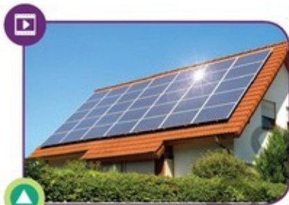
Figure 11.13 Solar panels harness energy from the Sun
