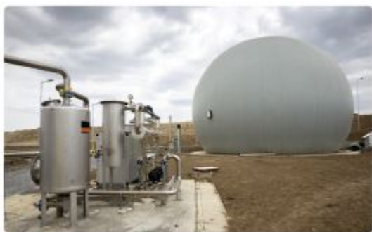
Natural gas tank
