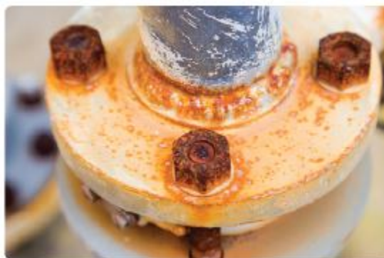
Corrosion is slow process
