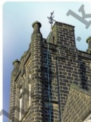
7.22 Lightning conductor on a school tower. The conductor consists of a metal strip, usually copper, of very low resistance connected to the ground below. A good connection to the ground is essential and is made by burying a large metal plate deep in the earth
