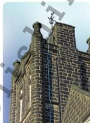
7.17 Lightning conductor on a school tower. The conductor consists of a metal strip, usually copper, of very low resistance connected to the ground below. A good connection to the ground is essential and is made by burying a large metal plate deep in the earth
