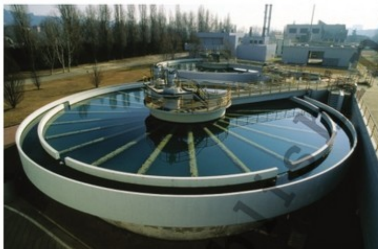
Figure 11.24 Flocculation and settling stage for purifying drinking water at a water works
