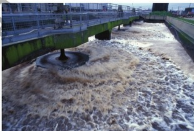
Figure 11.17 Secondary sewage treatment
